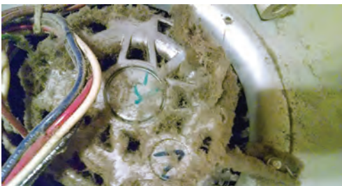
A dirty, inefficient blower caused by air bypass from a 1" filter.
