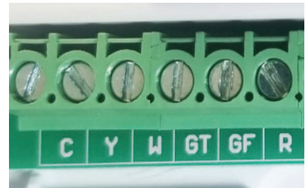
FIGURE 23: Thermostat and Air Handler Terminal on FAVC (Rotated 90°)
